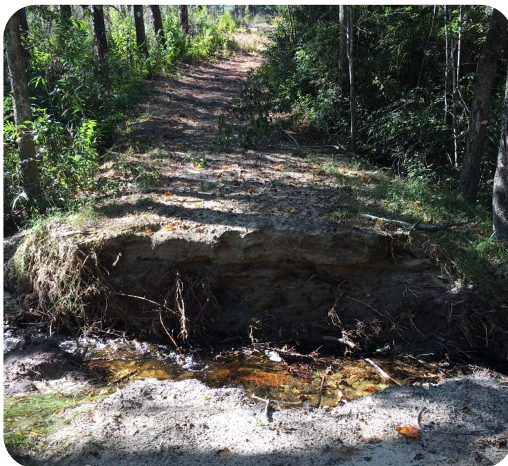
THE PIPE AT REFUGIO CROSSING WAS WASHED AWAY BY OCTOBER STORM
