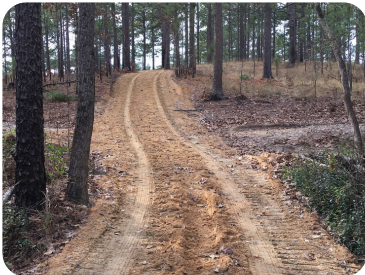
HOMESITE HILL WASHOUT REPAIR, LAWYER CROSSING
